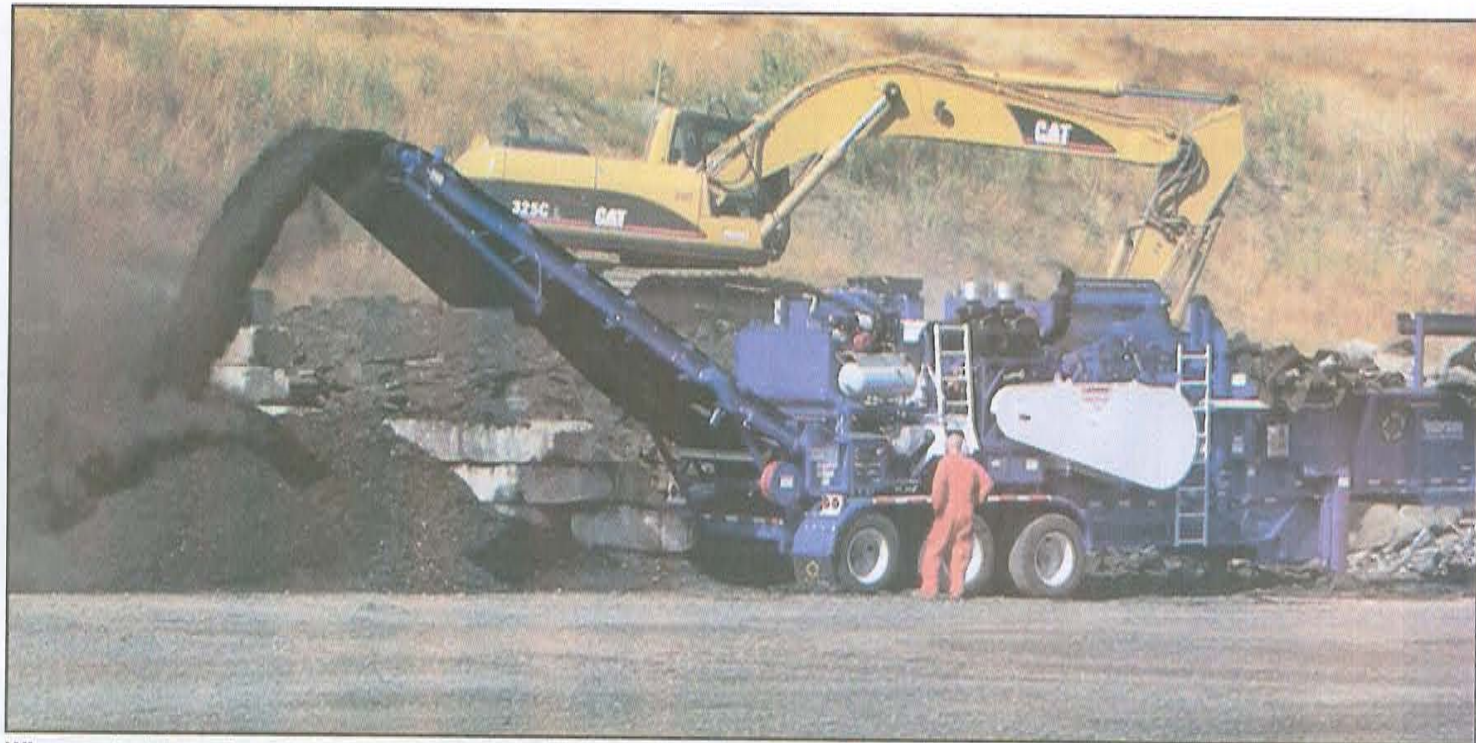
When material needs to be ground for recycling, Soiland looks to leased or contracted equipment to process the material. Here, asphalt shingle material is being ground for use in RAS asphalt.
